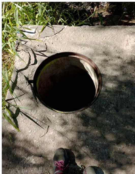
Descarga Emisario Portal o Shopping
